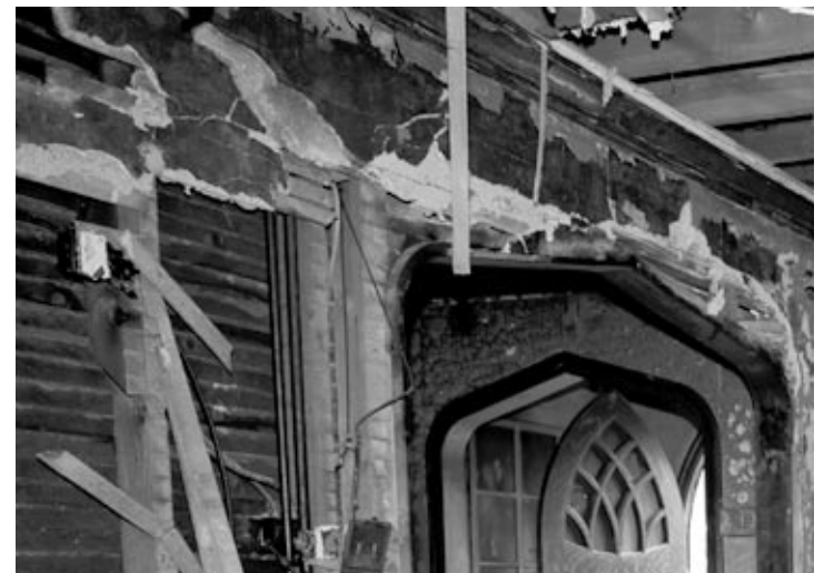
torn apart ★ The Migliazzos completely gutted their house during construction after a fire rendered the structure unstable. Photo SUBMITTED
